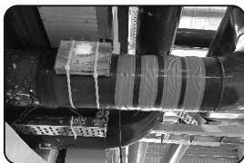
Central AC Plant (PVR Cinema)
